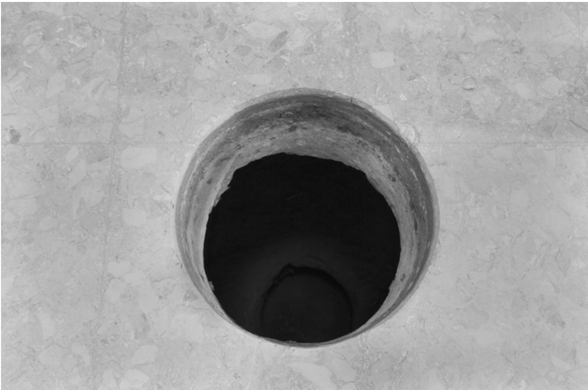
Il tempietto , view of the holes in the floor slab and in the ground, Rome, 2005, photo: Claudio Abate.
